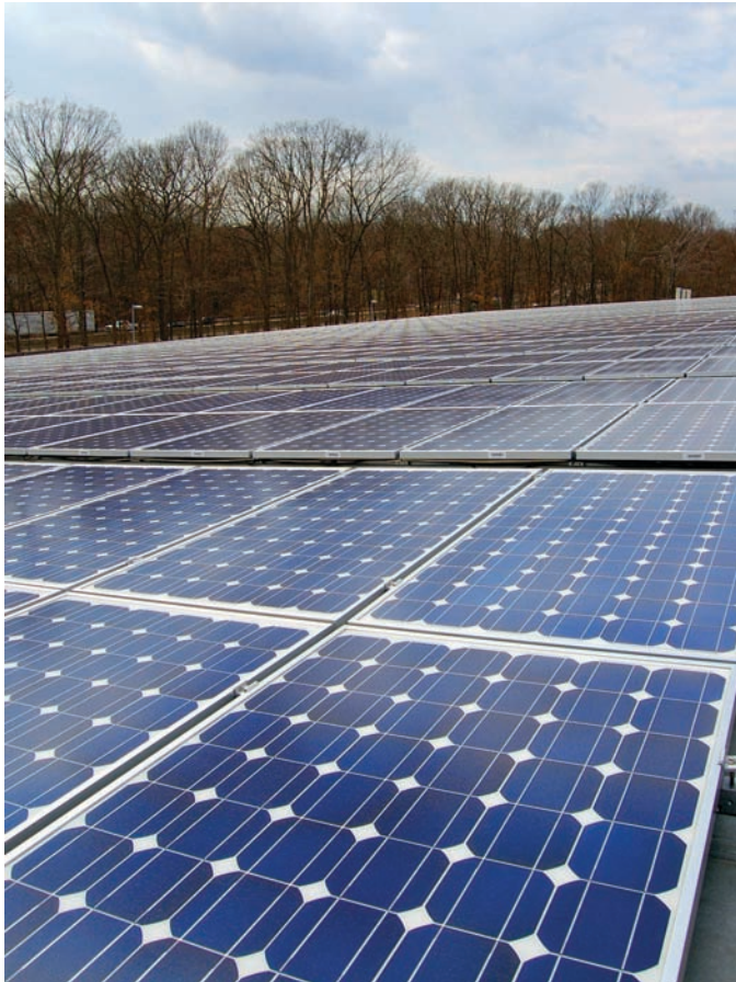
1,760 PV panels, 308kW Solar electric system - 282 tons of CO 2 generation avoided
