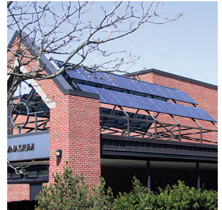
Spire Solar Systems provided PV services for all Chicago Partnership projects.
