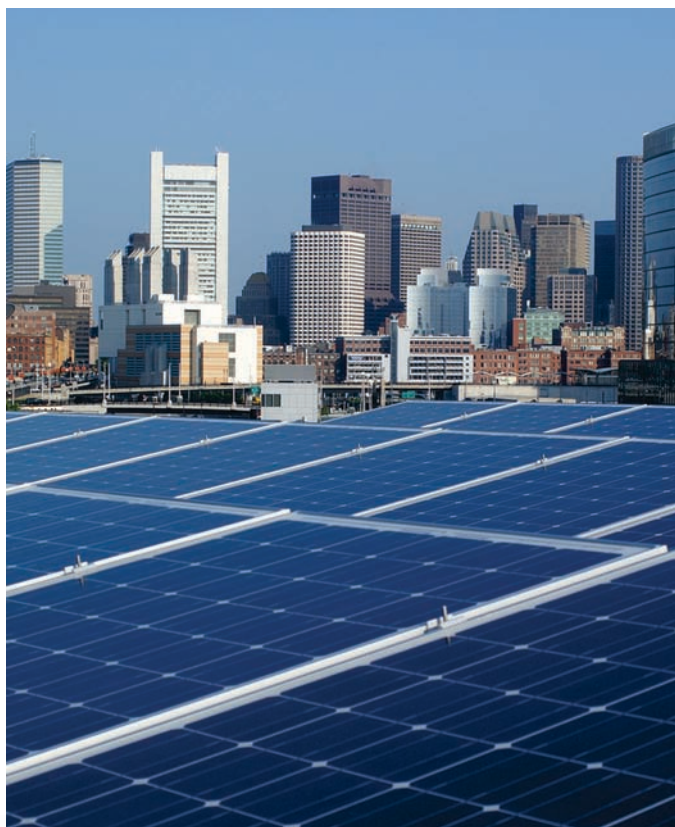
Largest PV installation in Boston, MA (USA)
